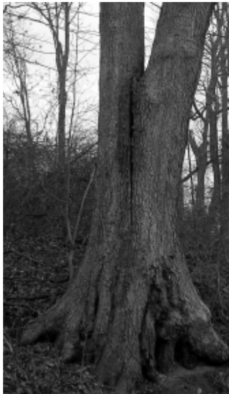
A branch junction with a crack extending vertically down from the “vee” of the main attachment may present a serious potential for harm.
